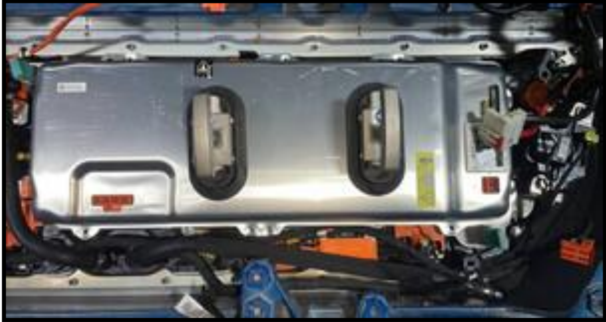
The DC-DC converter is located in the Penthouse of the Tesla battery. It is liquid cooled and shares space with the charge controller and other HV electronics
